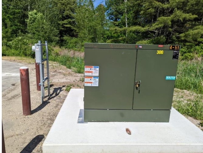
Figure 9 Dedicated Transformer for BEB Chargers at 13 Pomerleau St.
