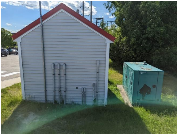
Figure 10 Saco TC Electrical Hut and Generator
