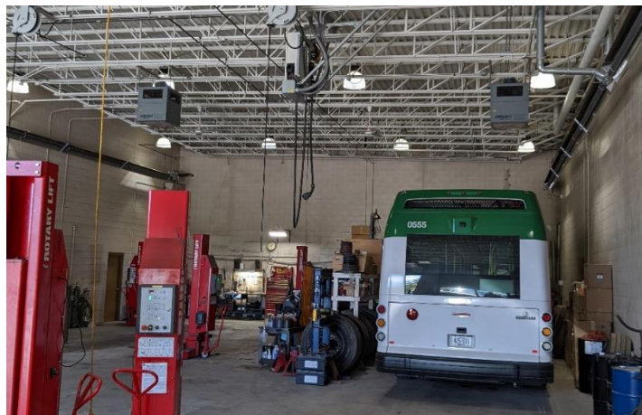
Figure 5 13 Pomerleau St Facility with DC Fast Chargers
